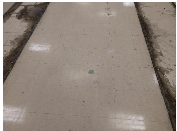
Photo #12 View of one of two previous soil-gas probe locations within the interior of the site building.
