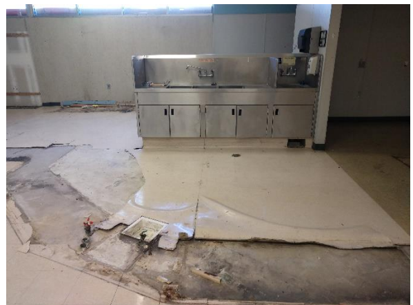
Photo #6 View of a previous sink area within the interior of the site.
