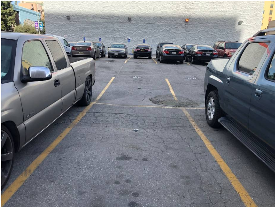
A low spot in the asphalt was observed centrally on the Subject Property.
