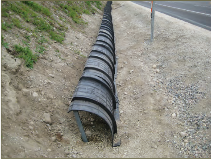
Photo 42. ACO fencing on highway near, Oliver, B.C. © R. Guse
