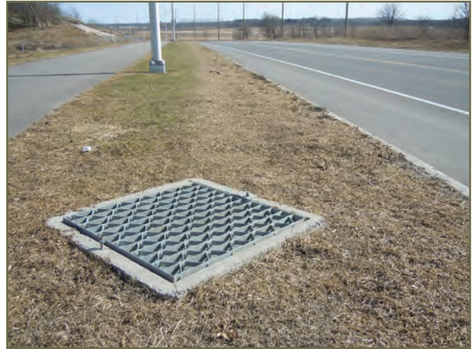
Photo 28. Open grate skylight in median on Terry Fox Extension, Ottawa, Ontario. © D. Seburn
