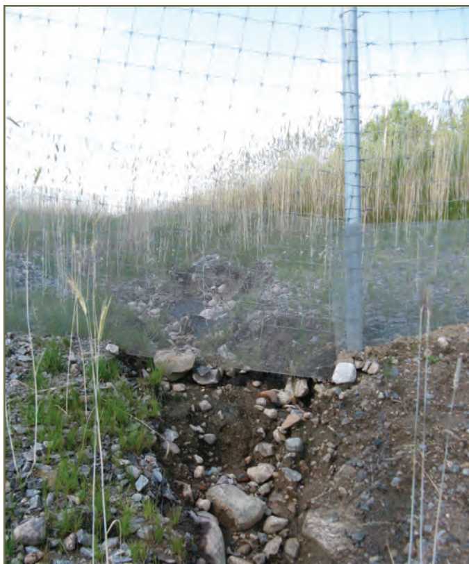
Photo 50. Fence with gap at bottom due to erosion from water draining under fence © K. Gunson
