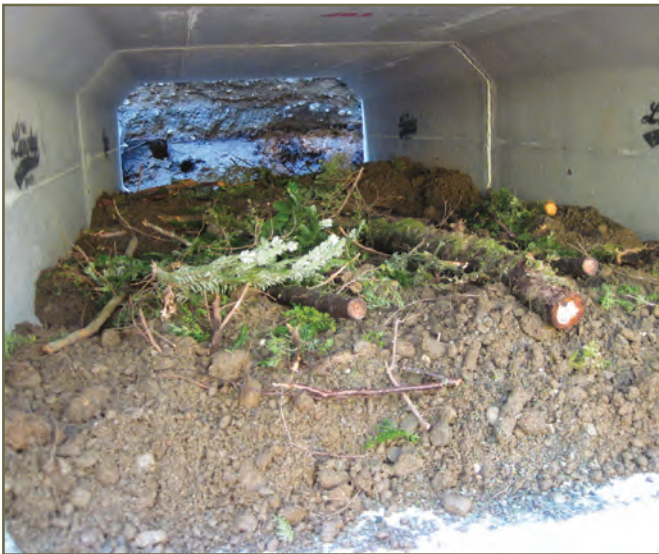
Photo 13. Soil and branches inside tunnel bottom, Ucluelet, B.C. ©Barb Beasley
