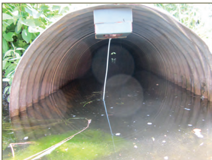
Photo 66. Camera securely fastened to top of culvert; note difficult to capture animals when water in culvert or tunnel. © K. Gunson
