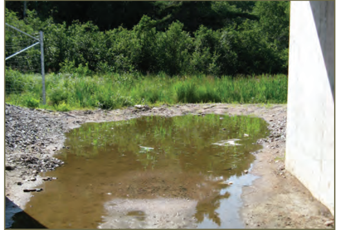
Photo 31. Water accumulation at tunnel entrance. © K. Gunson
