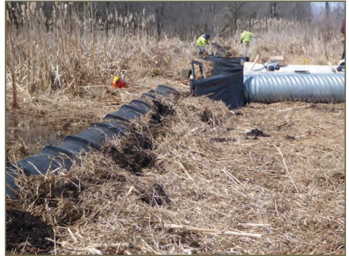
Photo 49. Backfill along ACO wildlife fence that can provide an escape ramp for animals on the roadside of the fence © V. D'elia
