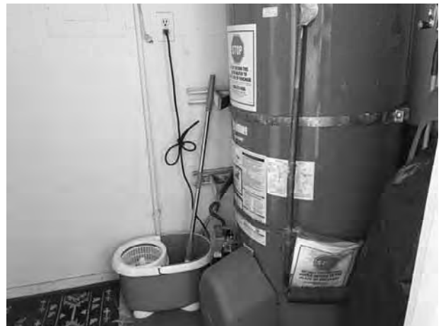
12. View of a typical boiler, in building A.
